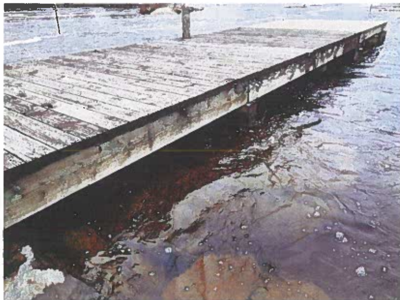
Existing dock showing condition of decking and proximity of bedrock support
