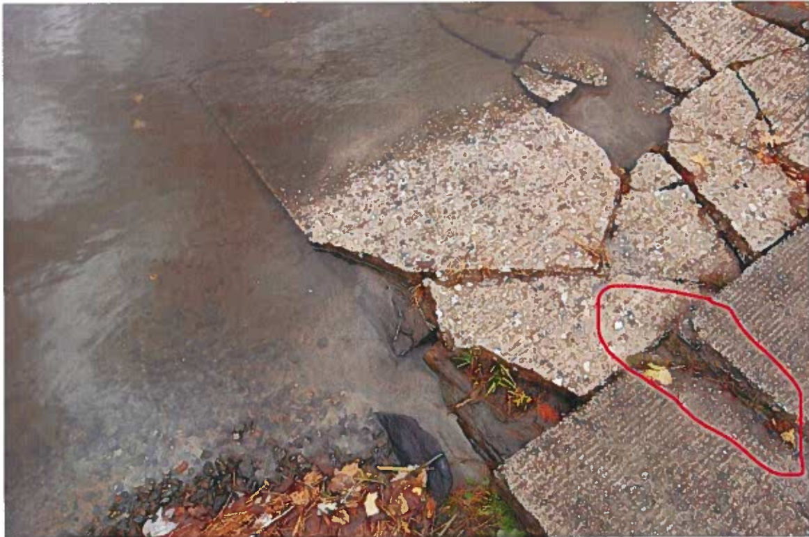
Portion of broken slab showing exposed welded wire mesh and extent of deterioration
