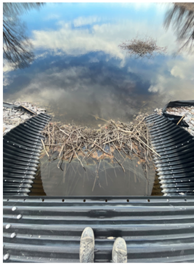
Figure 3 - Culvert Facing Northwest – Beaver dam obstruction
