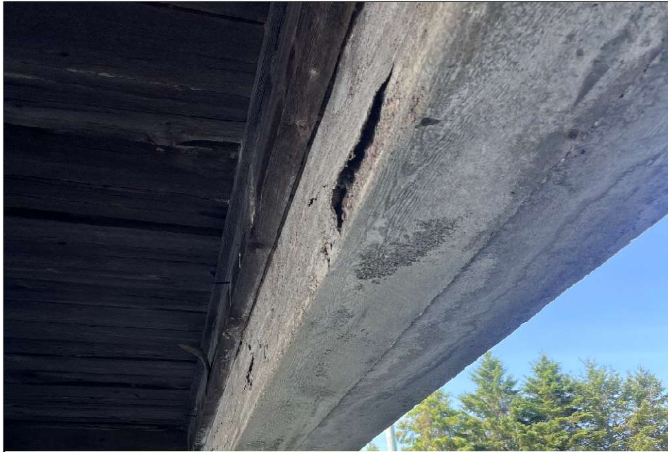
Photo 3: Delamination on Girder
