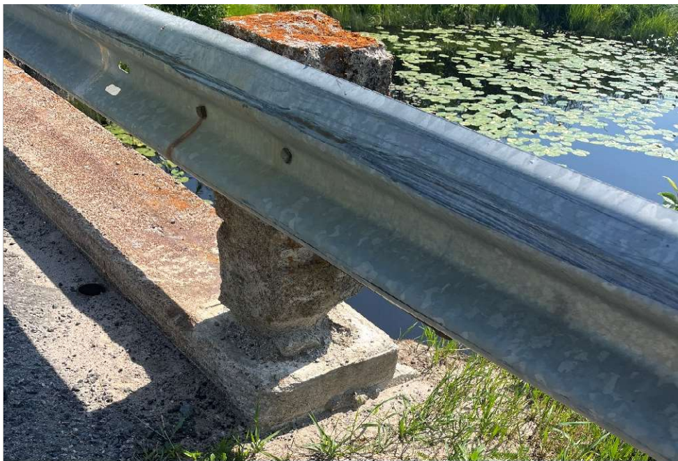
Photo 4: Disintegration of Railing Balustrade
