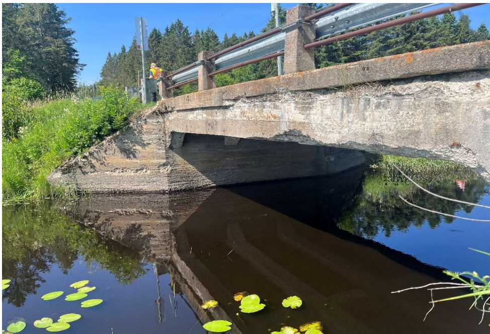
Photo 2: Elevation view of the structure showing exposed rebar and damage to girders
